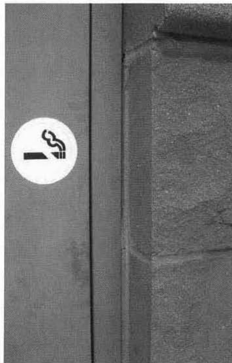
Photo No. 5: North façade grade level exit door – no sealant in joint between door frame and cast stone building base.
