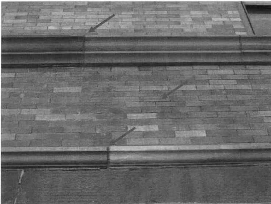
Photo No. 2: South façade brick spandrel and sandstone horizontal bands – typical area of open mortar joints at brick spandrel areas and occasionally cracked and open mortar joints at sandstone bands.
