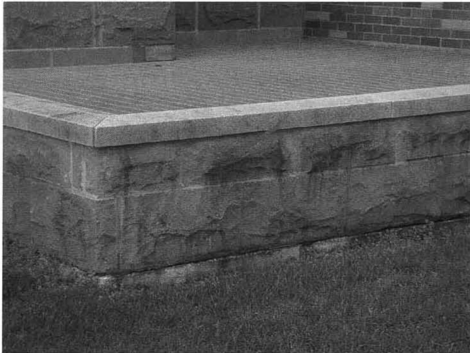
Photo No. 2: North façade cast stone wall with cap at equipment intake/exhaust – organic staining.
