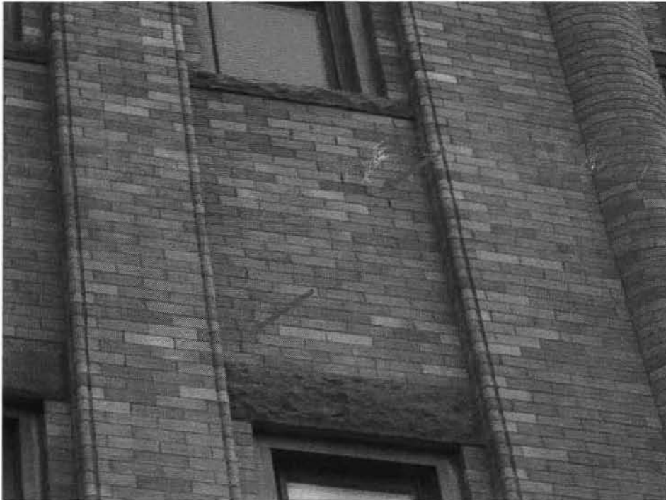
Photo No. 1: West façade spandrel area – typical area of step cracking with cracked brick and open mortar joints.
