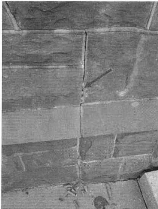
Photo No. 4: South façade sandstone building base – limited open joints at sandstone masonry.
