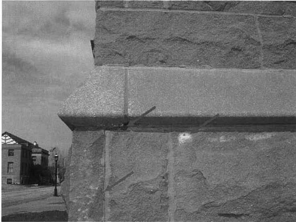
Photo No. 1: North façade cast stone base and horizontal band – minor cracked and open mortar joints and efflorescence. Note: Cast stone was used on the new addition to simulate cut natural stone.
