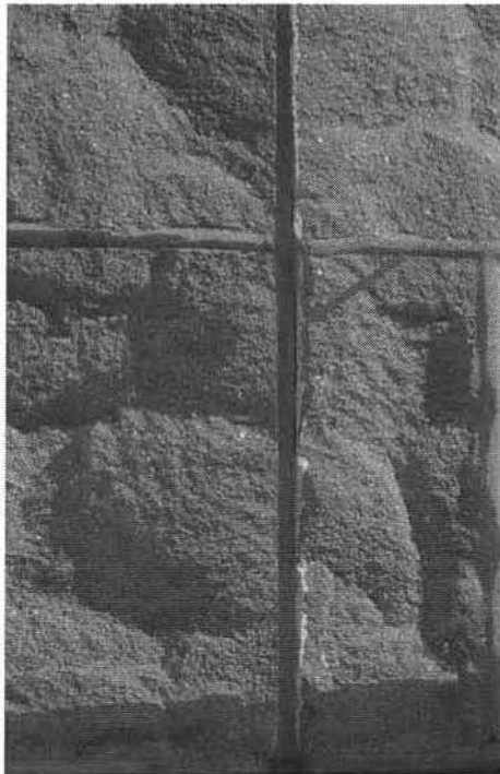
Photo No. 4: South façade cast stone building base – expansion joint sealant failure.
